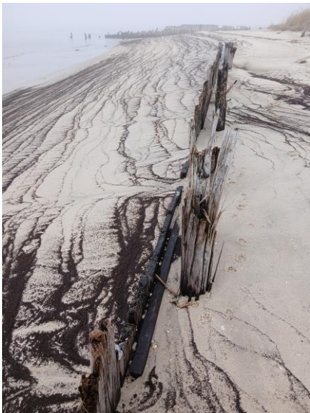
Horizontal derelict bulkhead (rubble).
